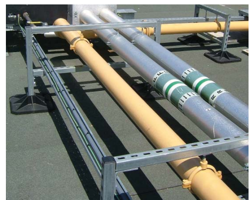
Big Foot H frame supporting pipework (both installations for Essex County Council Buildings, Chelmsford, Essex)
